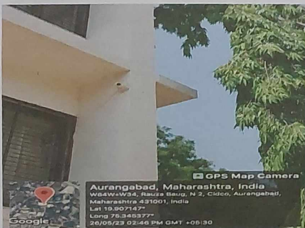
CCTV Cameras at Entrance Building
